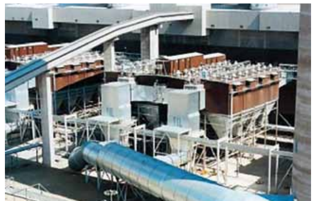
Eskom Majuba coal power plant
